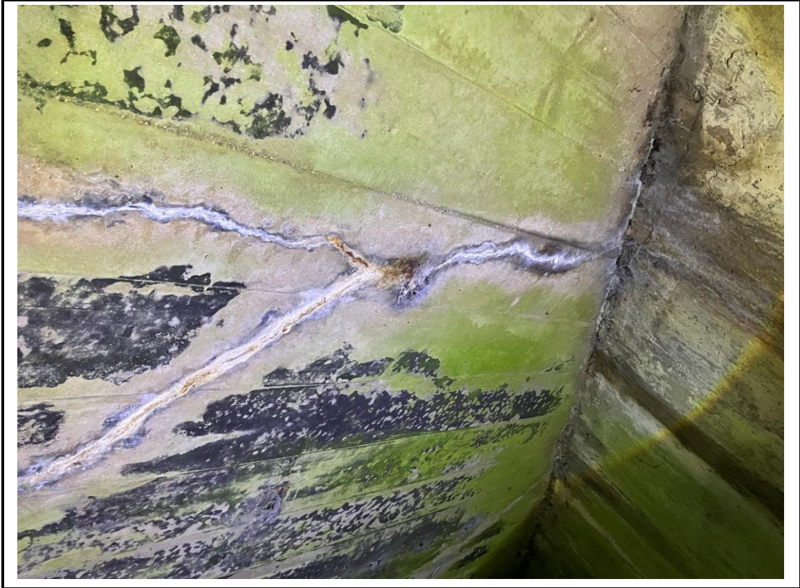
1717_P11_2024 Bridge soffit - Diagonal and longitudinal cracks
