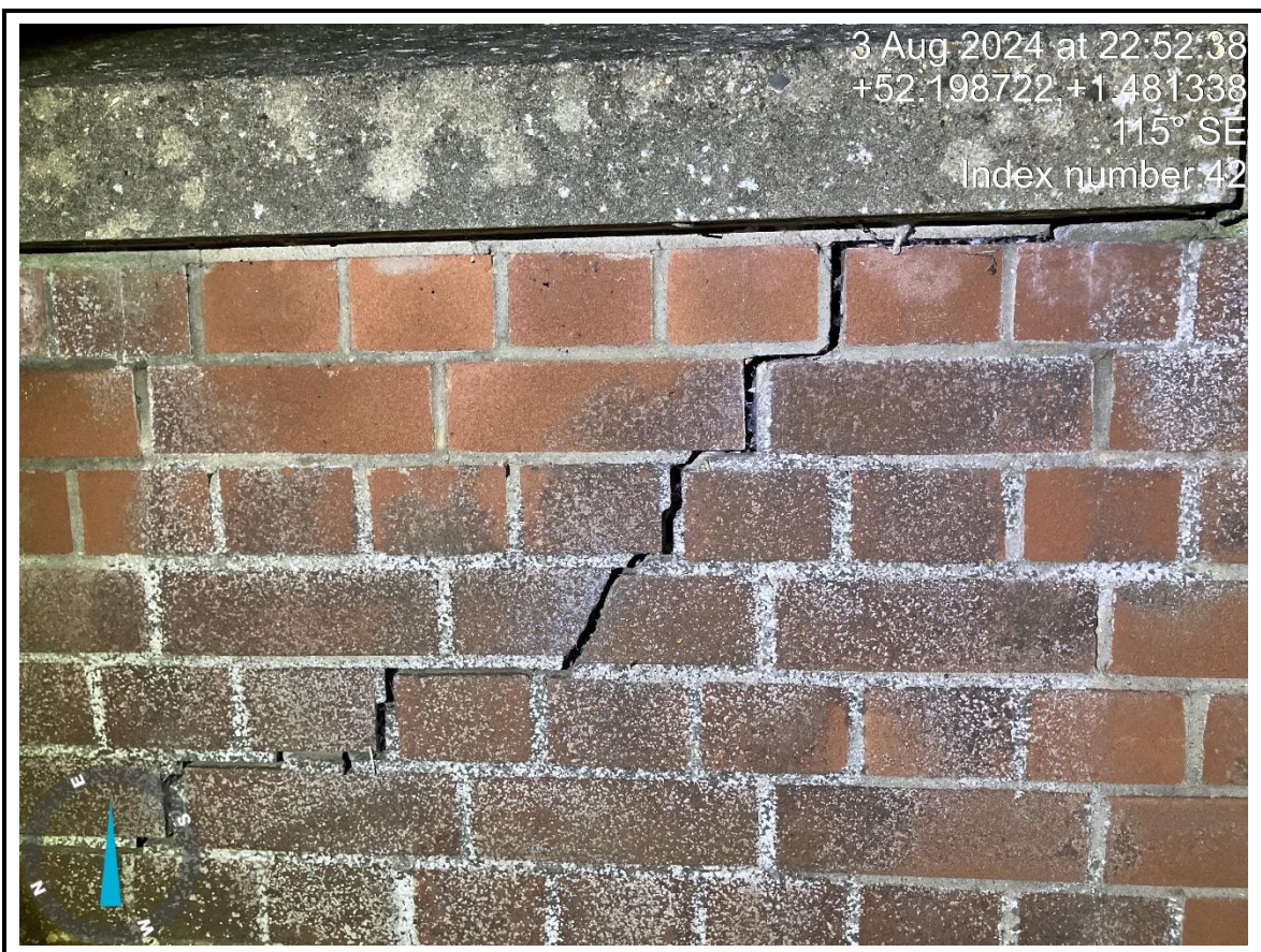
1717_P33_2024 South parapet - Diagonal parapet crack (<10mm)
