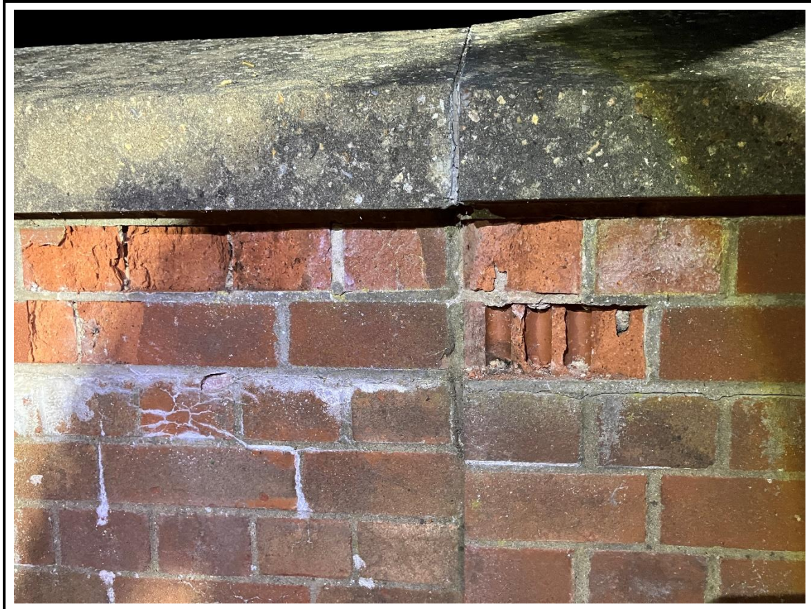
1717_P40_2024 North parapet - Brick spalling & hairline cracks
