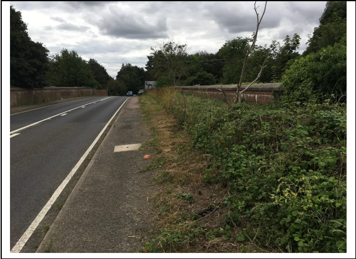
1717_P43_2024 North footway - Footway surfacing and vegetation growth (July 2023)
