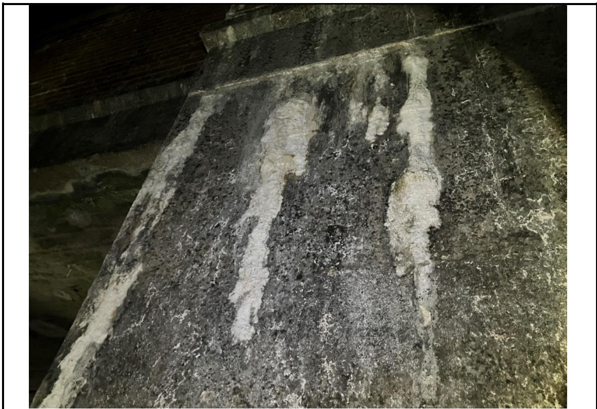
1717_P54_2024 Northwest wingwall - Active saline leachate deposits (<15mm)
