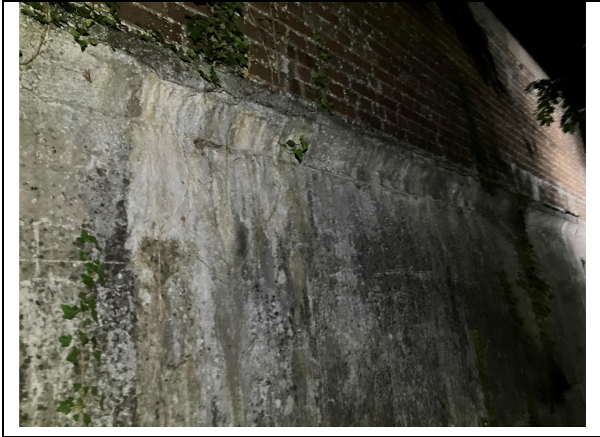
1717_P57_2024 Northeast wingwall - Active saline leaching
