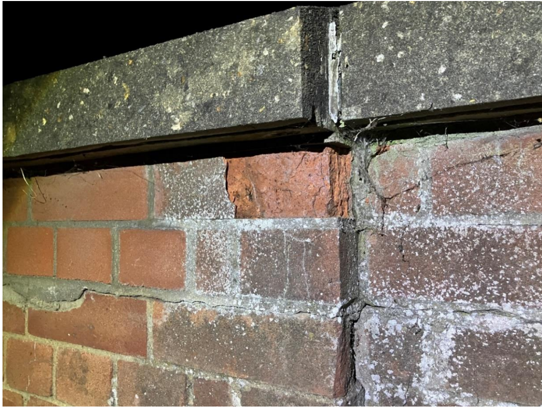
1717_P34_2024 South parapet - Brick spalling (10mm deep) & horizontal hairline crack
