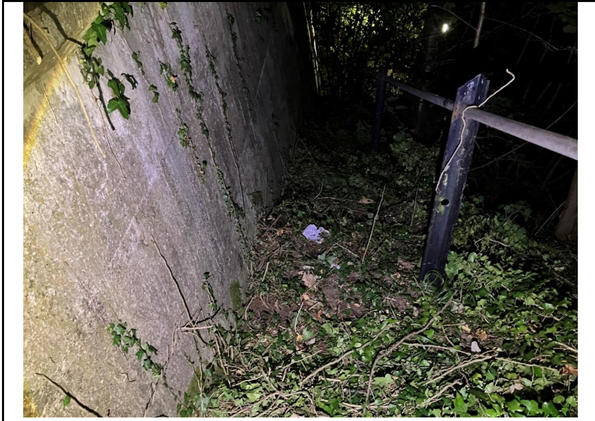
1717_P45_2024 Southwest wingwall - Leaching & vegetation growth
