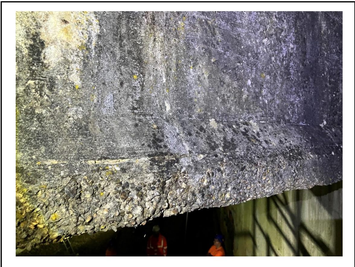
1717_P12_2024 North deck edge – Minor concrete spalling
