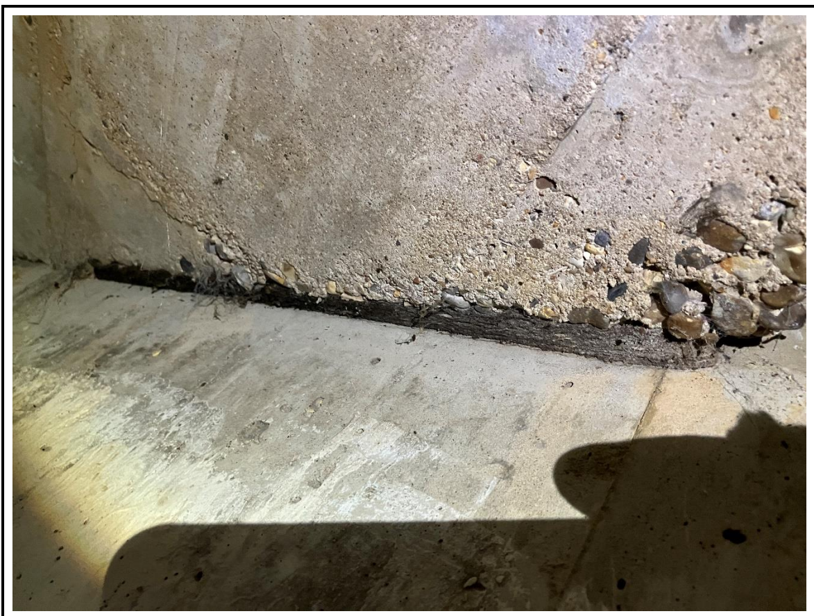
1717_P16_2024 Abutment/soffit interface – Deteriorated filler board
