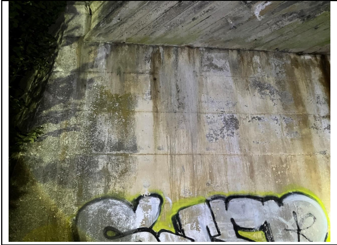
1717_P17_2024 West abutment – Saline leaching and corrosion staining
