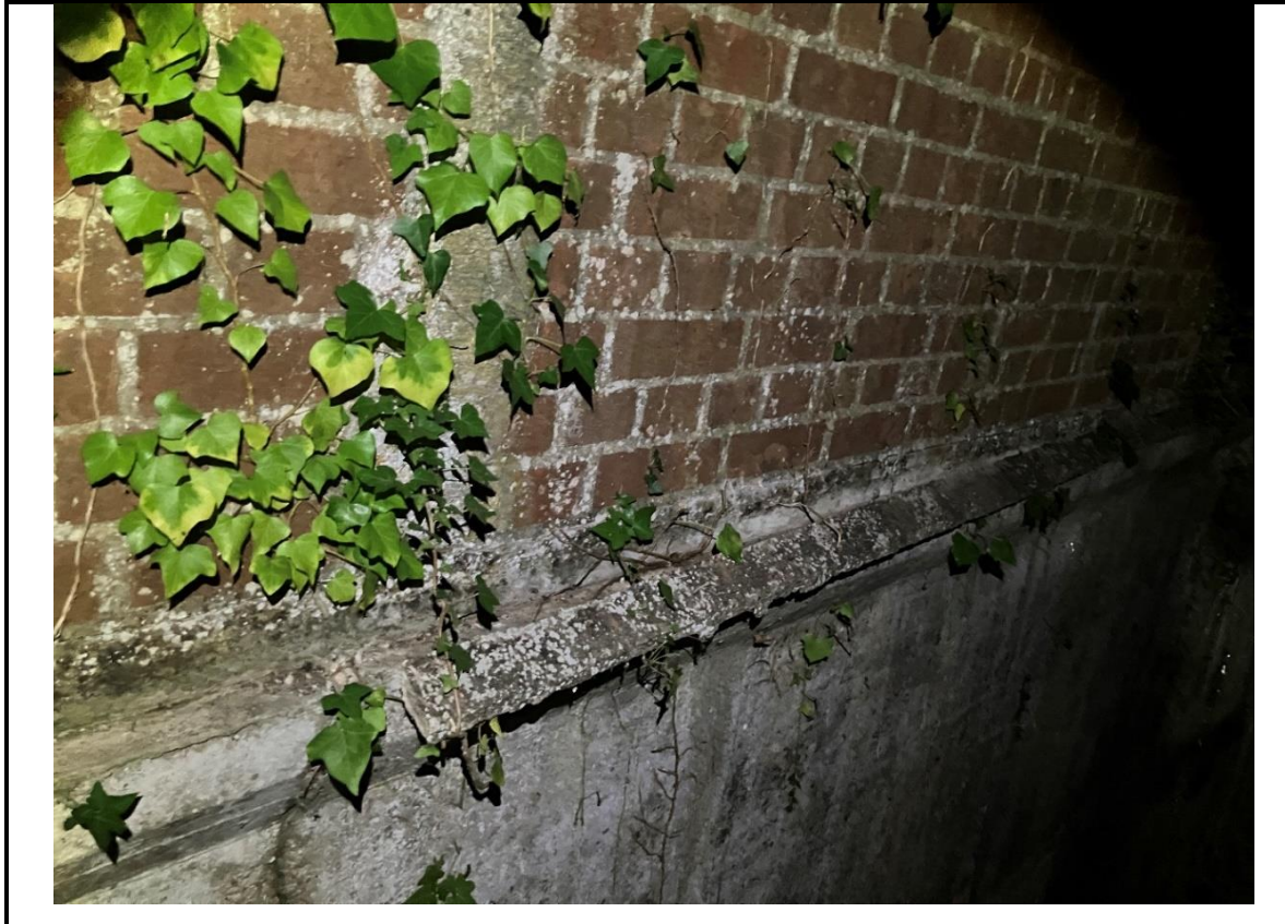
1717_P58_2024 Northeast wingwall - Mortar fillet peeling off
