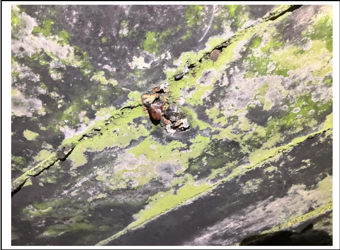
1717_P15_2024 Bridge soffit – Exposed corroded threaded bar
