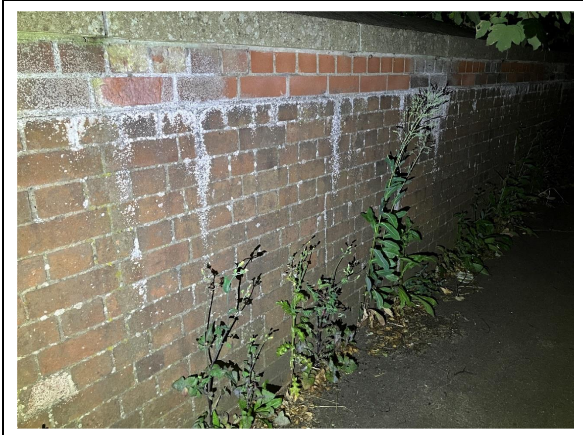
1717_P36_2024 South parapet - Minor vegetation growth & historic leaching
