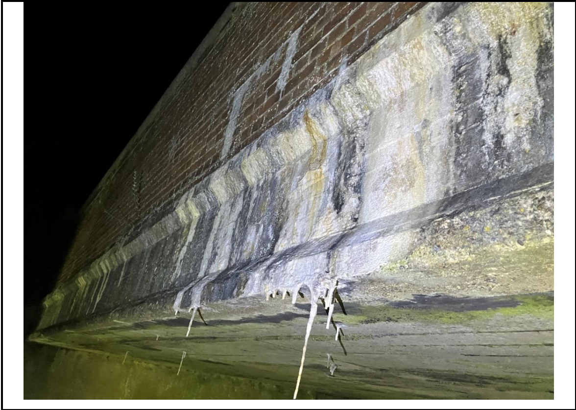
1717_P13_2024 North deck edge - Leachate deposits (<5mm thick) with stalactite build up (also to soffit between beam construction joints)
