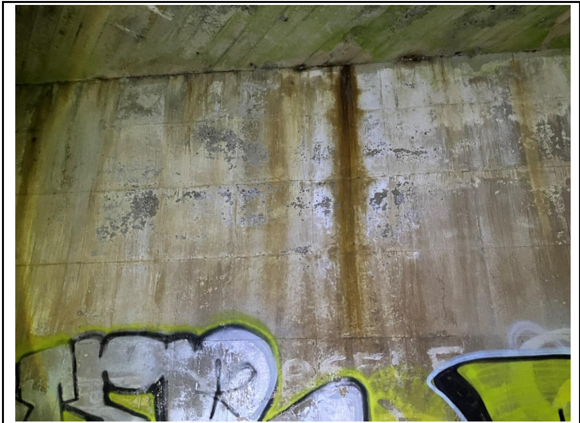
1717_P20_2024 West abutment - Saline leaching and corrosion staining
