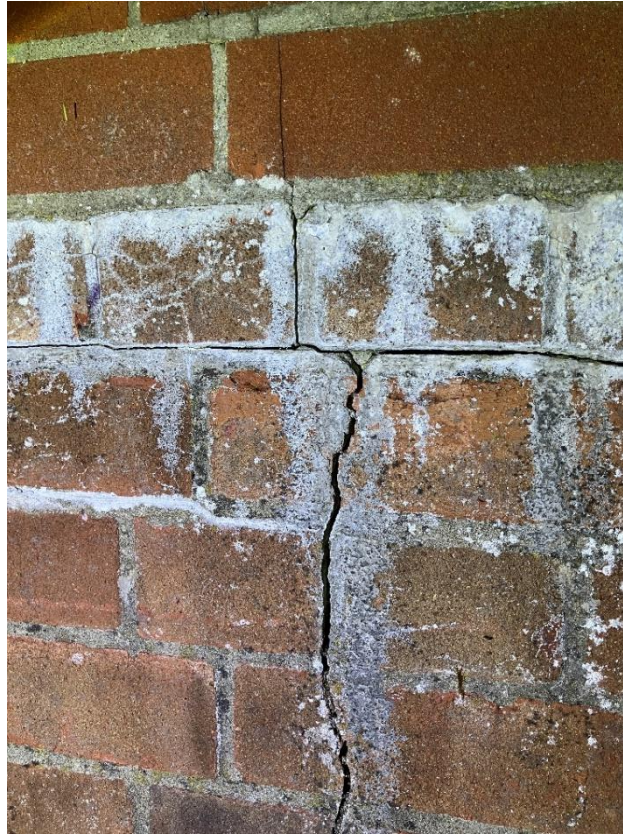
1717_P38_2024 North parapet - Vertical crack (<2.5mm), horizontal crack (<3mm) & leaching
