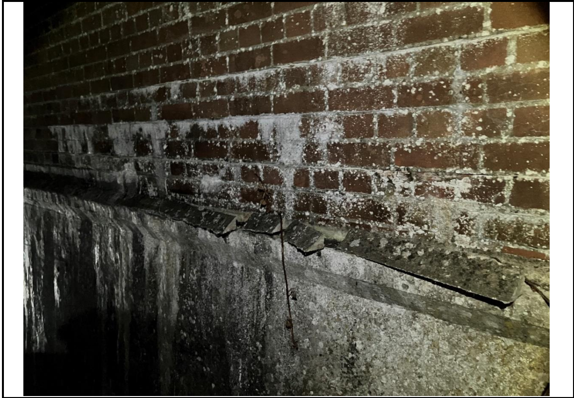
1717_P55_2024 Northwest wingwall - Mortar fillet peeling off
