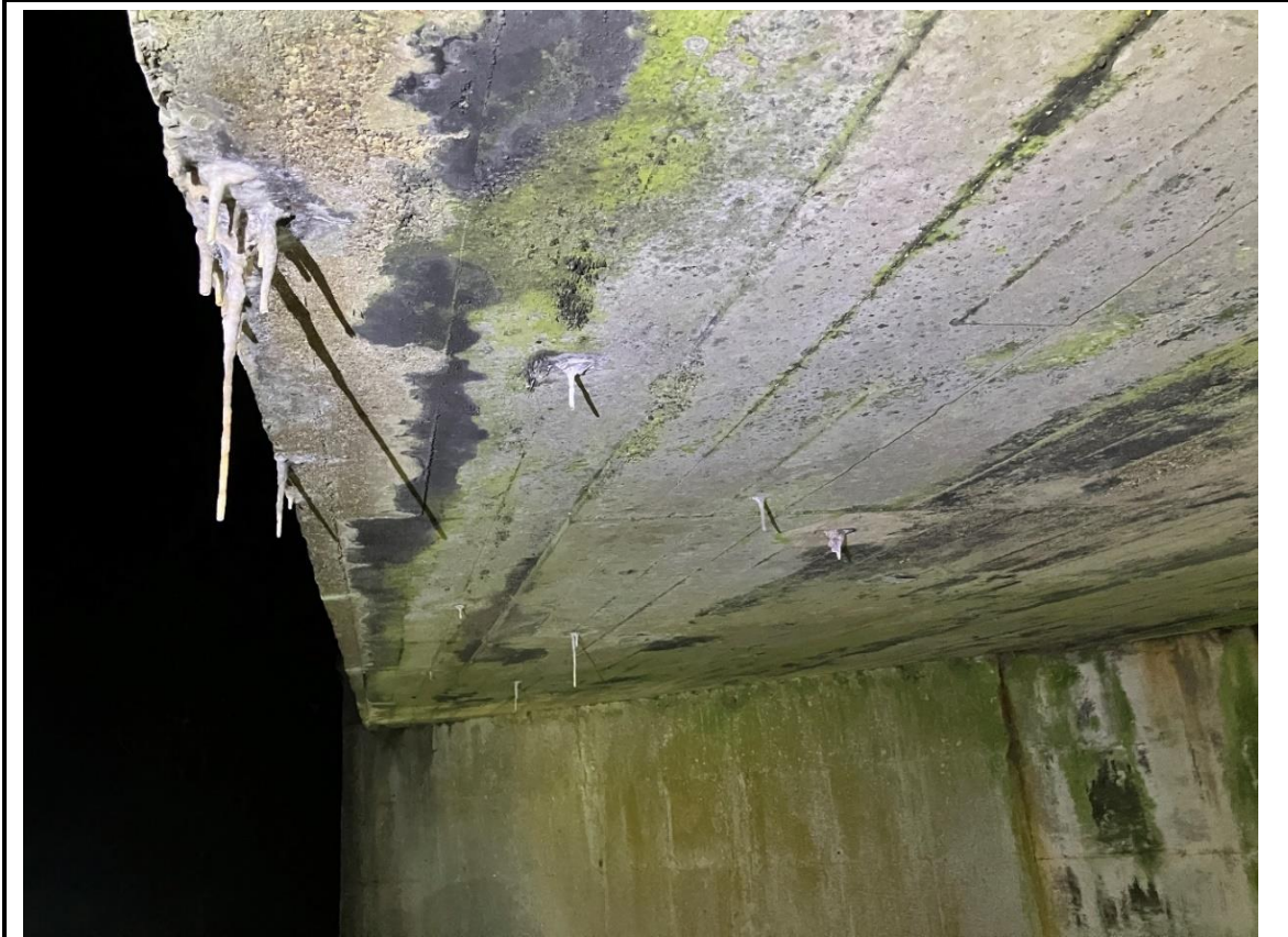
1717_P30_2024 Bridge soffit/Edge beam (North footway) - Stalactite formation (<200mm)
