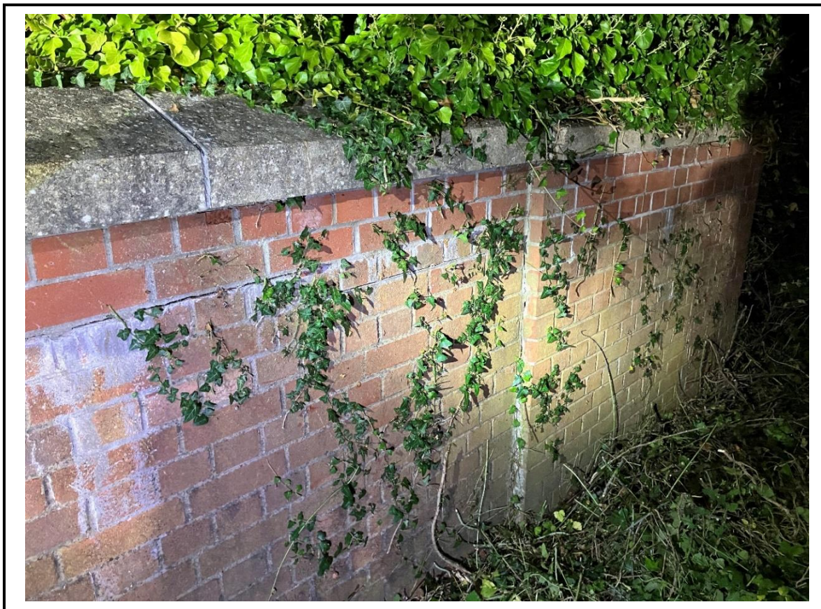
1717_P37_2024 North parapet – Horizontal crack (<2mm), footpath & vegetation growth
