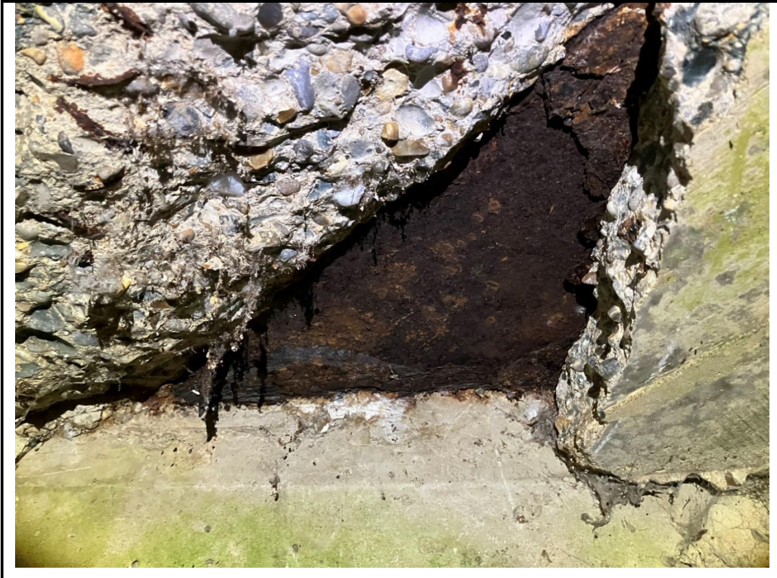
1717_P5_2024 West abutment/soffit interface – Exposed corroding steel I beam (75mm Cover)
