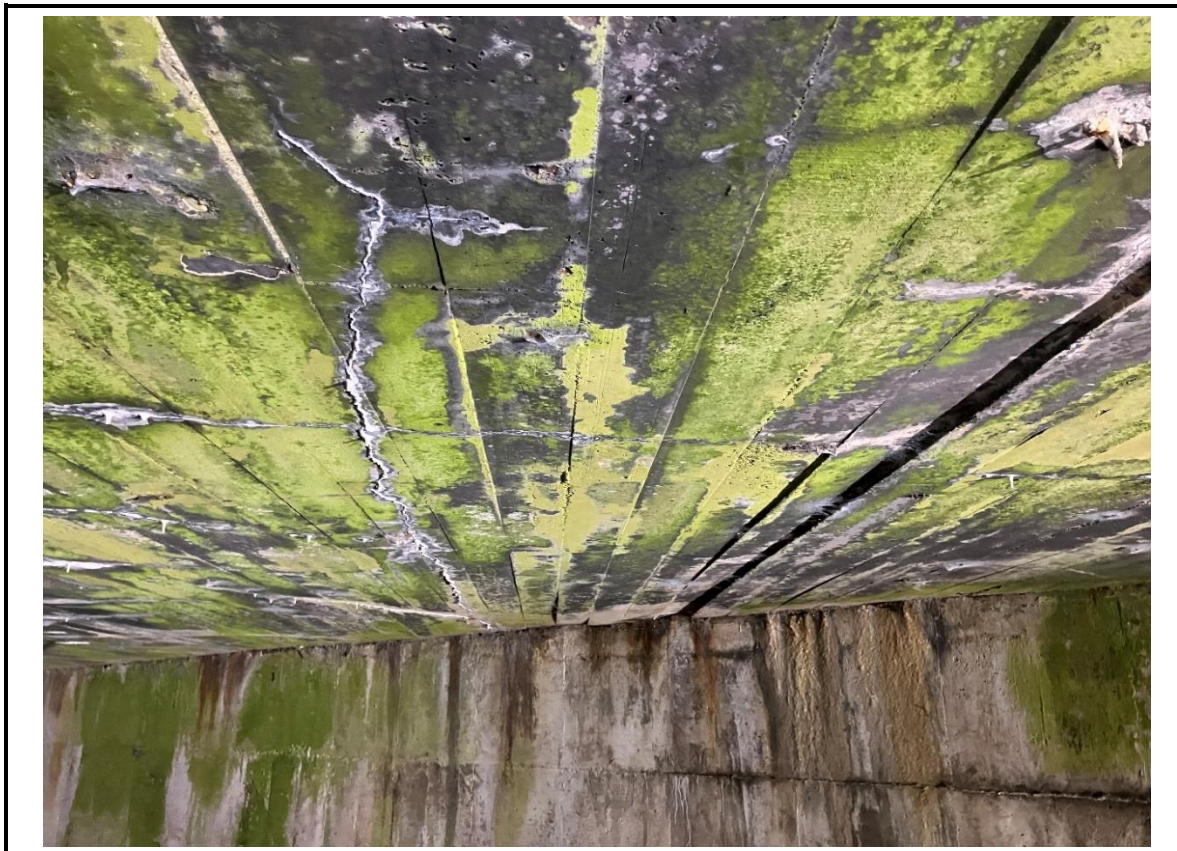
1717_P22_2024 East abutment - Saline leaching and corrosion staining
