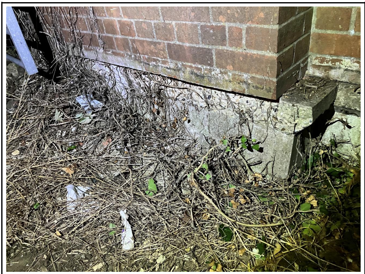
1717_P48_2024 Southwest pilaster - Concrete spalling (<75mm) below pilaster
