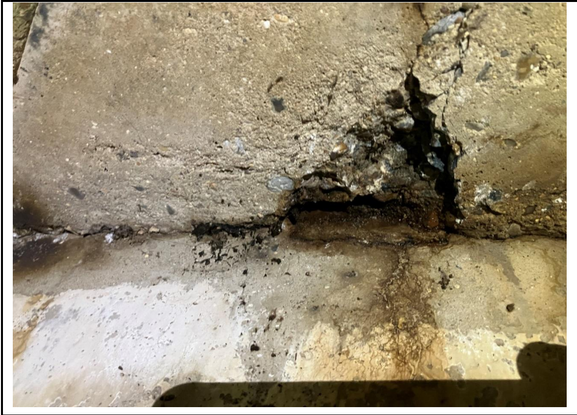
1717_P7_2024 West abutment/soffit interface - Partial spalling & exposure of steel beam
