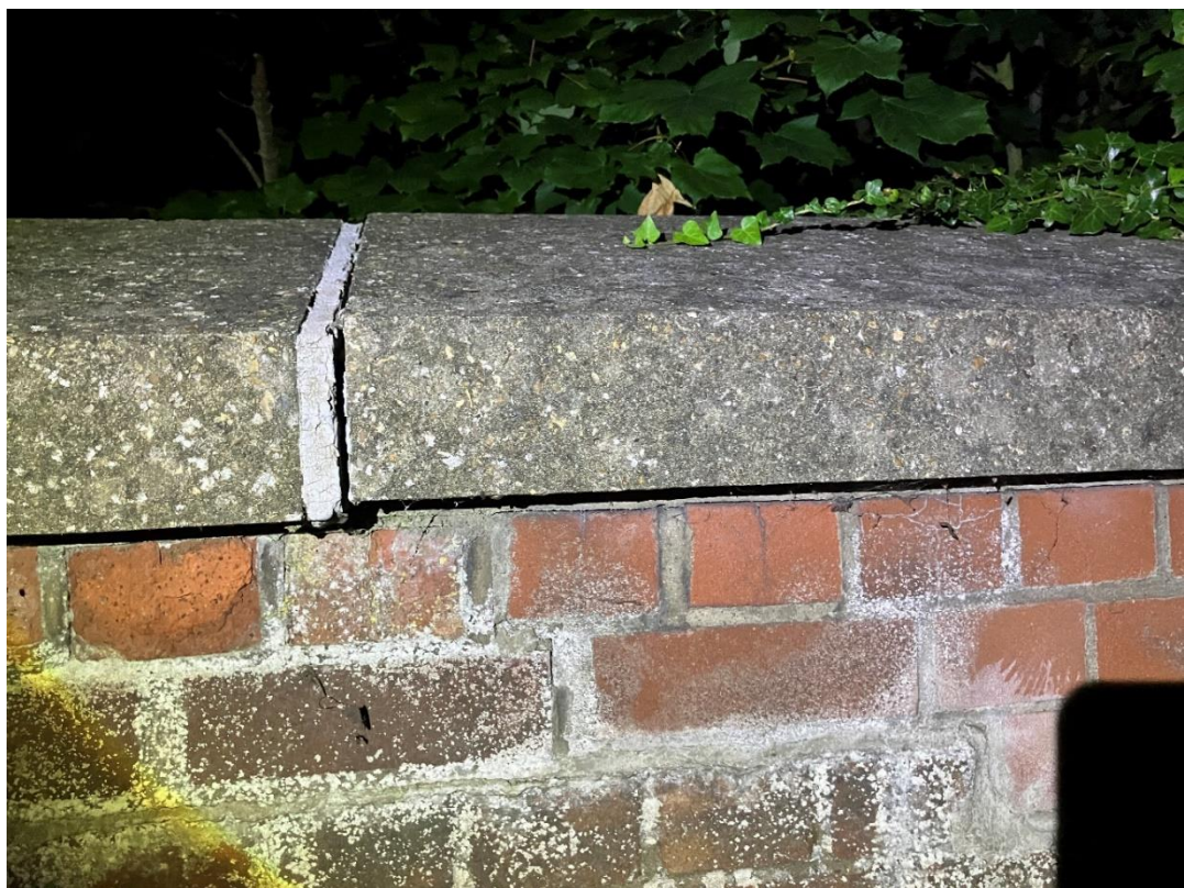
1717_P35_2024 South parapet – Displacement of parapet coping (<15mm) & repaired diagonal crack
